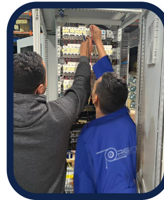
I/O Test check
