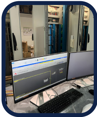
SCADA System in FAT
